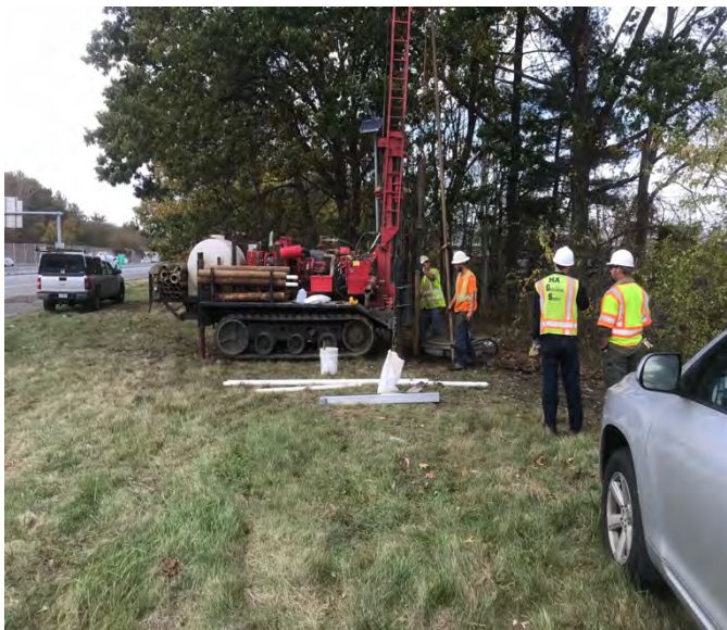
Installation of new monitoring well for the climate response network. Well is located in Wakefield along Route 128.
